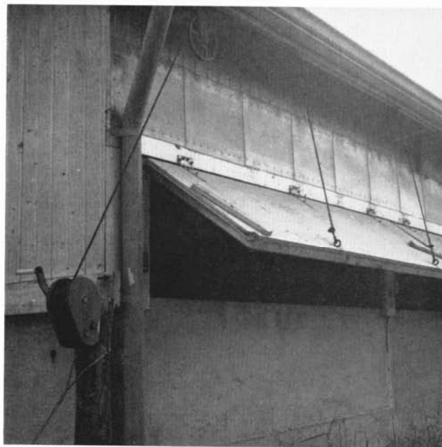
Fig. 25. Side doors allow additional air movement for summer ventilation.
