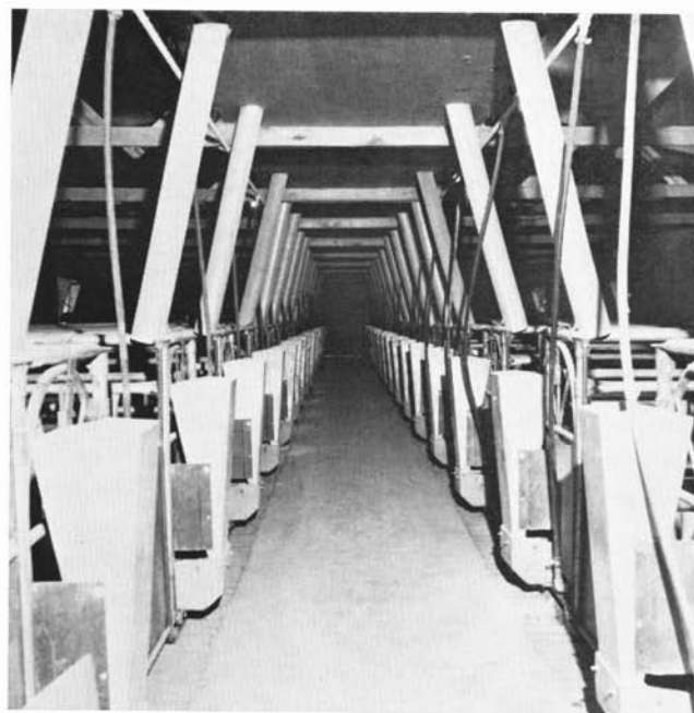
Fig. 26. Ventilation duct with individual air supply for each sow during the summer.
