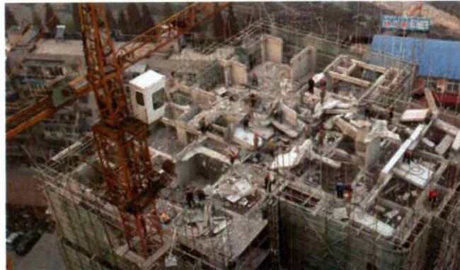
high rises in China are often torn down after 20-30 years, generating a huge amount of waste upon demolishing
