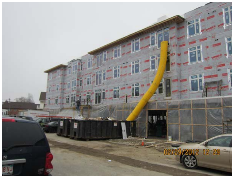
Figure 12 - All modules and systems are connected
