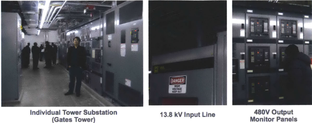
Figure 47: Human-scale references for a variety of electrical systems contained in the Stata Center electrical substations
