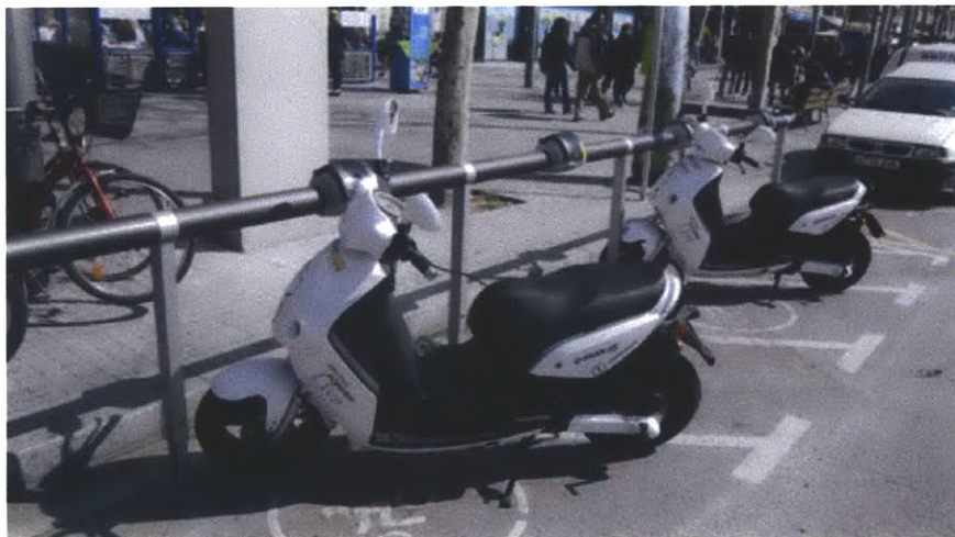
Figure 8: Electric Motorcycle Charging Stations in Barcelona, designed by Mobecpoint. These stations employ a standard charge plug and do not incorporate a docking or locking mechanism.
