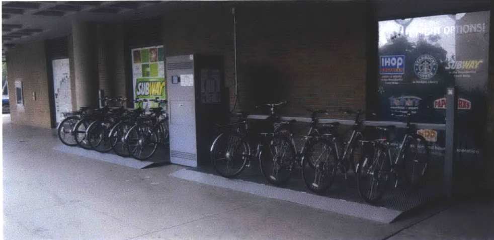
Figure 7: An electric bicycle sharing station at University of Tennessee, Knoxville. The central unit is a battery recharger and vending machine that is connected to electrical infrastructure via a central conduit, visible on the brick wall. This station utilizes battery swapping rather than an integrated charging and docking system.
