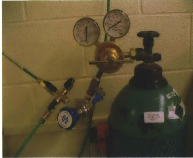
Figure 13: Photo of the Nitrogen Gas System with lines to the accumulator and fill tank [29].
