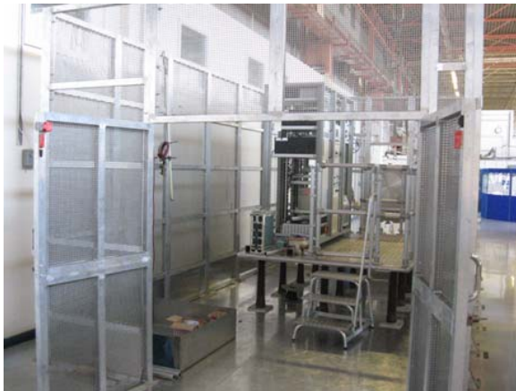
Figure 2: The high voltage cage and 65 kV high voltage platform.
