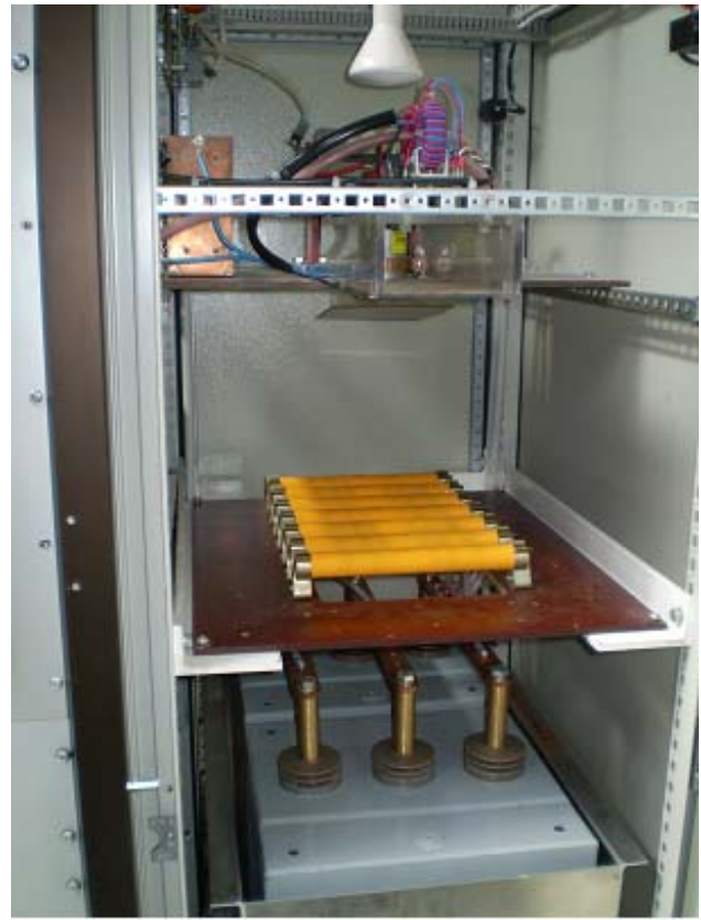
Figure 3: The replacement second harmonic anode power supply capacitors.
