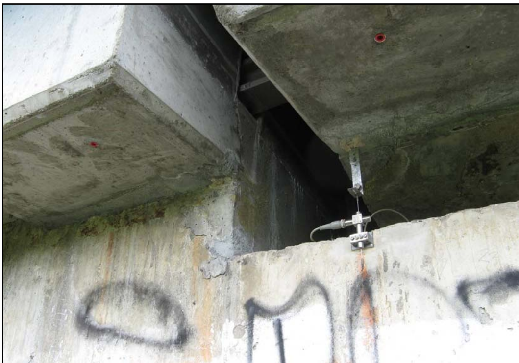
Fig. 130 - Measuring the vertical displacement expansion joints in section R111 of pier 10 on the left edge of the bridge
