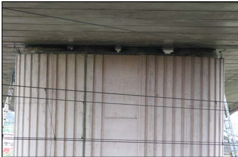
Fig. 132 - View of the sensors placed in sections R81 and R82 on pillars No. 8
