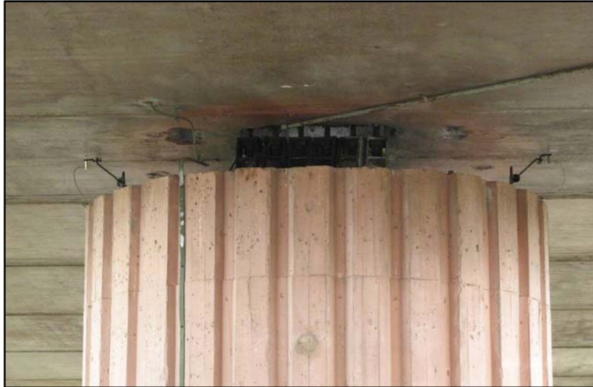
Fig. 131 - View of the sensors placed in sections R92 and R93 in Pillar No. 9
