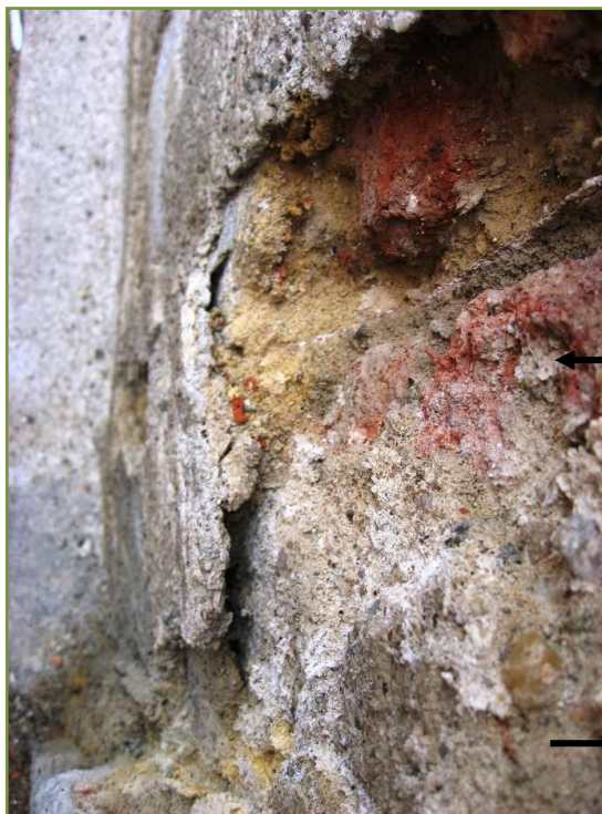
Figure 8: Detachment of plaster due to the subflorescence
