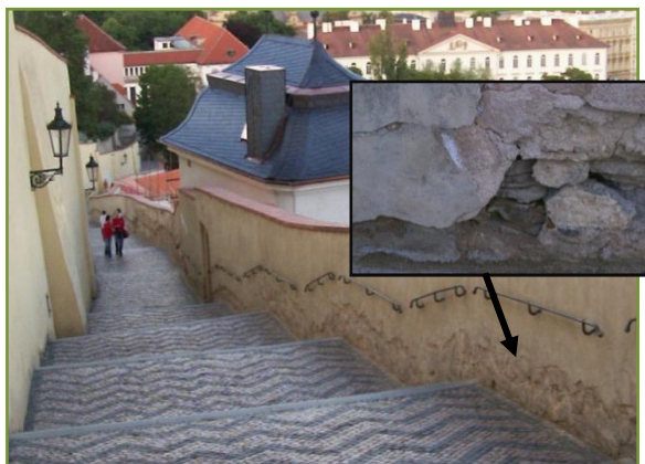
Figure 5: Damage due to salt crystallization (Prague, Czech Republic)
