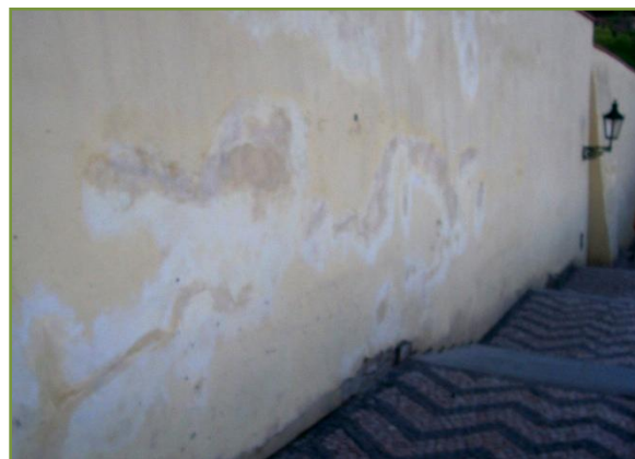
Figure 6: Salt efflorescence on a wall (Prague, Czech Republic)
